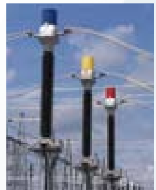
300kV, oil insulated current transformers
