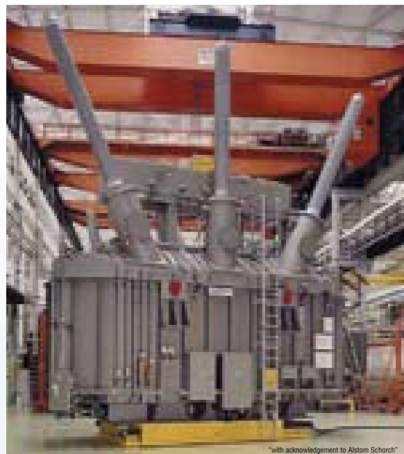
420kV & 123kV oil insulated transformer bushings with composite insulators
