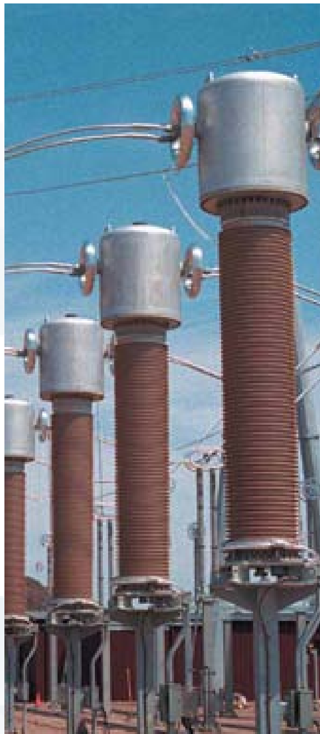
500kV, SF 6 insulated current transformers with composite insulators
