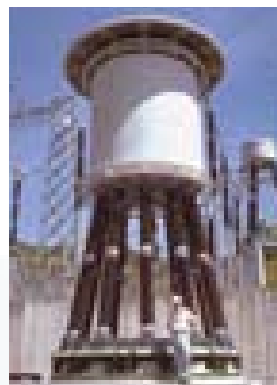
350kV HVDC smoothing reactor with seismic damping system
