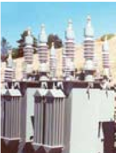
46kV oil insulated transformer bushings
