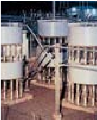
Thyristor controlled reactors in a static var compensator (SVC)
