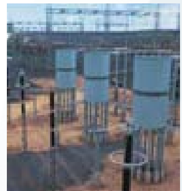
500kV, transmission bus tie reactor
