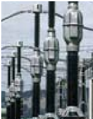
420kV, Oil insulated potential transformer
