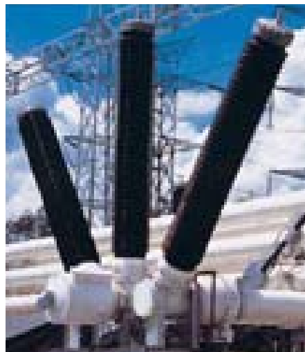
245kV, SF 6 to Air bushings
