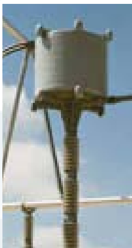
Epoxy resin impregnated/encapsulated line trap mounted directly on a coupling capacitor
