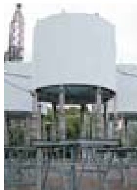
115kV, 30 ohm, series load flow reactors
