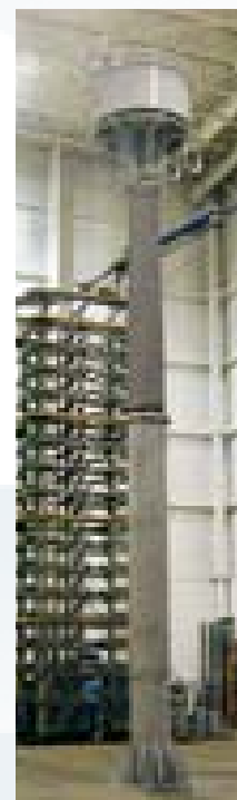
500kV line trap mounted onto a platform/composite foam filled insulated combination
