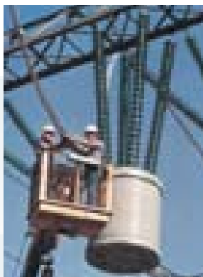
500kV suspension mounted line trap
