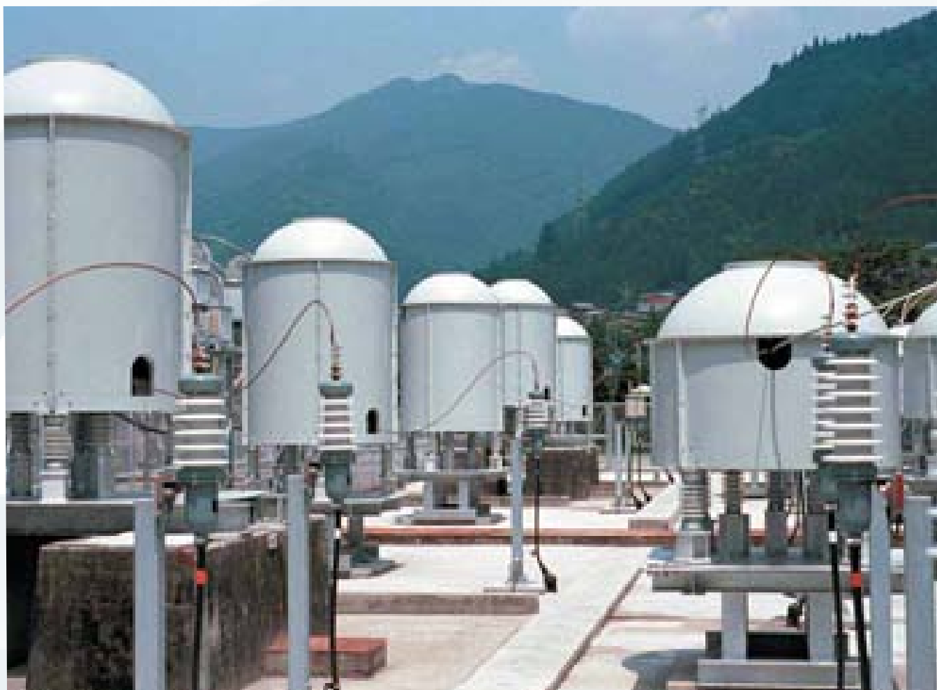
AC harmonic filter reactors with sound mitigation shields
