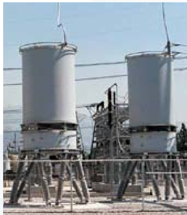
230KV, AC filter reactors with seismically designed support structures
