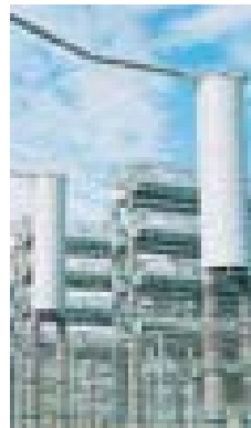
500kV, Capacitor reactors
