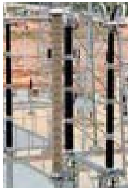
500kV, SF 6 insulated unit with composite insulator
