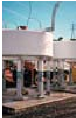
13.8kV, tertiary connected shunt reactors
